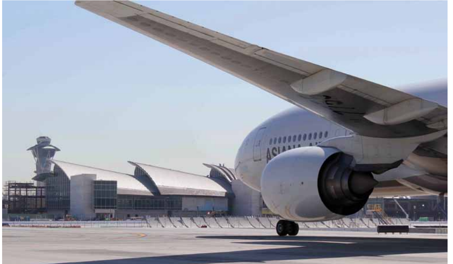
The construction of the new Tom Bradley International Terminal, which will provide Los Angeles with a world-class transportation facility, is expected to create 4,000 jobs over a three-year delivery schedule. Walsh Austin Joint Venture, the builder for the massive terminal at LAX, was recently recognized by the Los Angeles Minority Business Development Agency for its "Service to the People of Los Angeles." The project strives to dramatically improve ticketing, security checkpoints, and passenger lounges as well as expanding customs and immigration facilities. The improvement anticipates the terminal to process 4,000 passengers an hour, 30 percent more than its current capacity. Photo by Brian Williams.
